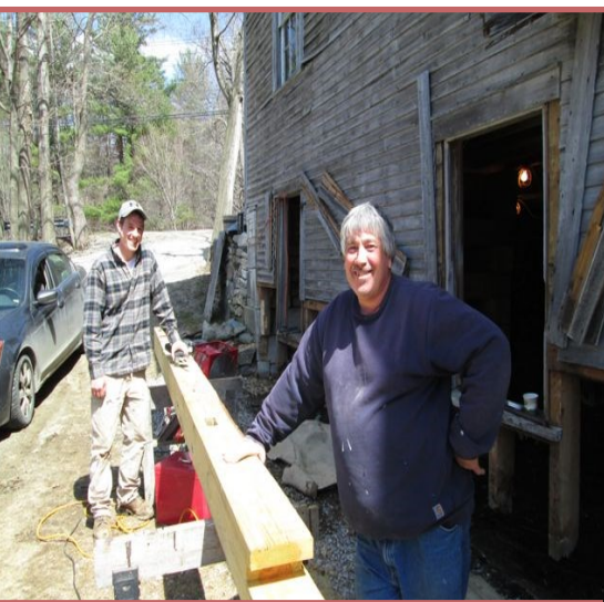
Steve Fisher and assistant, Justin Lourie, prepare to jack up the barn and repair sills and beams
